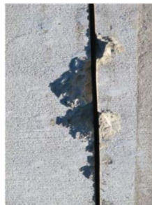
Bad shoe on early entry saw
