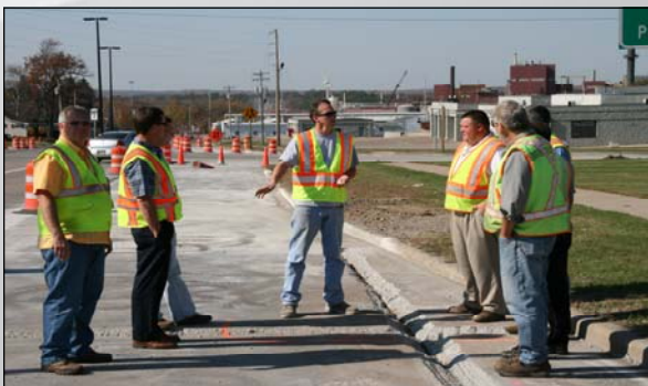
Picture of a ground out repair section: Tom Bonness Jr. of CPR, Inc. explains to the group the finer points of removals for partial depth repairs by the Vermeer wheel.
