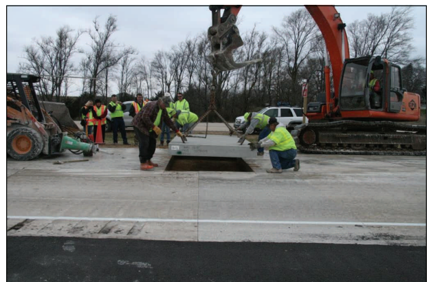
CPR, Inc. staff lowering the new slab into place. Retrofit dowel bars are installed immediately after the slab is in place.
