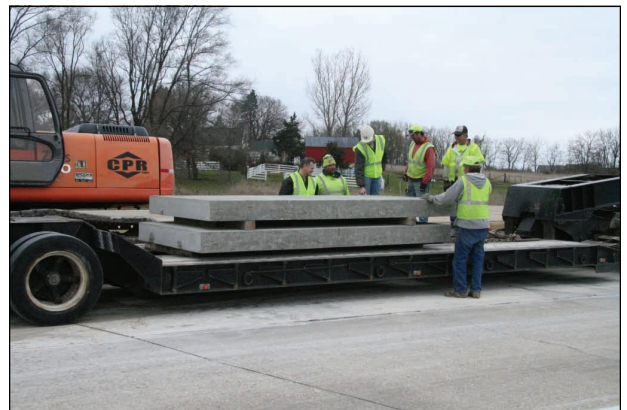
CPR, Inc and Mid-States Concrete Industries staff inspects the 6'x12' precast concrete slabs delivered to the USH 151 project.
